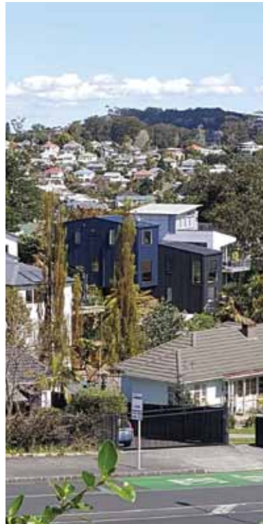
perches comfortably on low cost timber pole foundations that anchor into the rock 6m below ground.
