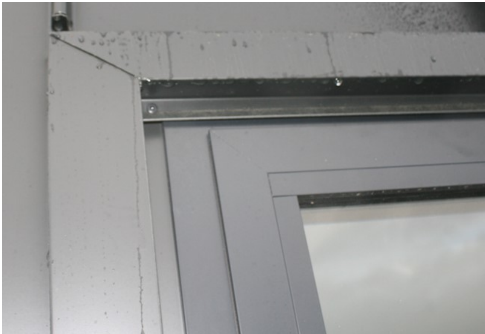
Using clipped flashings to minimise the use of rivets is a feature of a well-installed standing seam roof.
